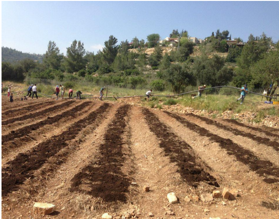
Installing the main water pipe, a donation by Netafim. Planting begins within days.
